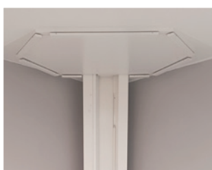
Fire seals for both levels
